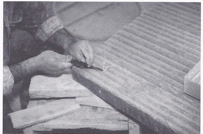
4 Excess glue at glue-line can be peeled away after mix takes its initial set—from five to fifteen minutes depending on temperature.
