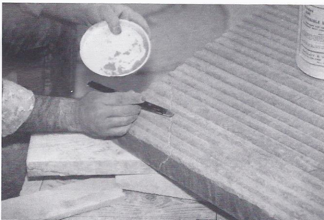
5 Minor "pluckouts" at glue-line can be covered with cementitious material.
